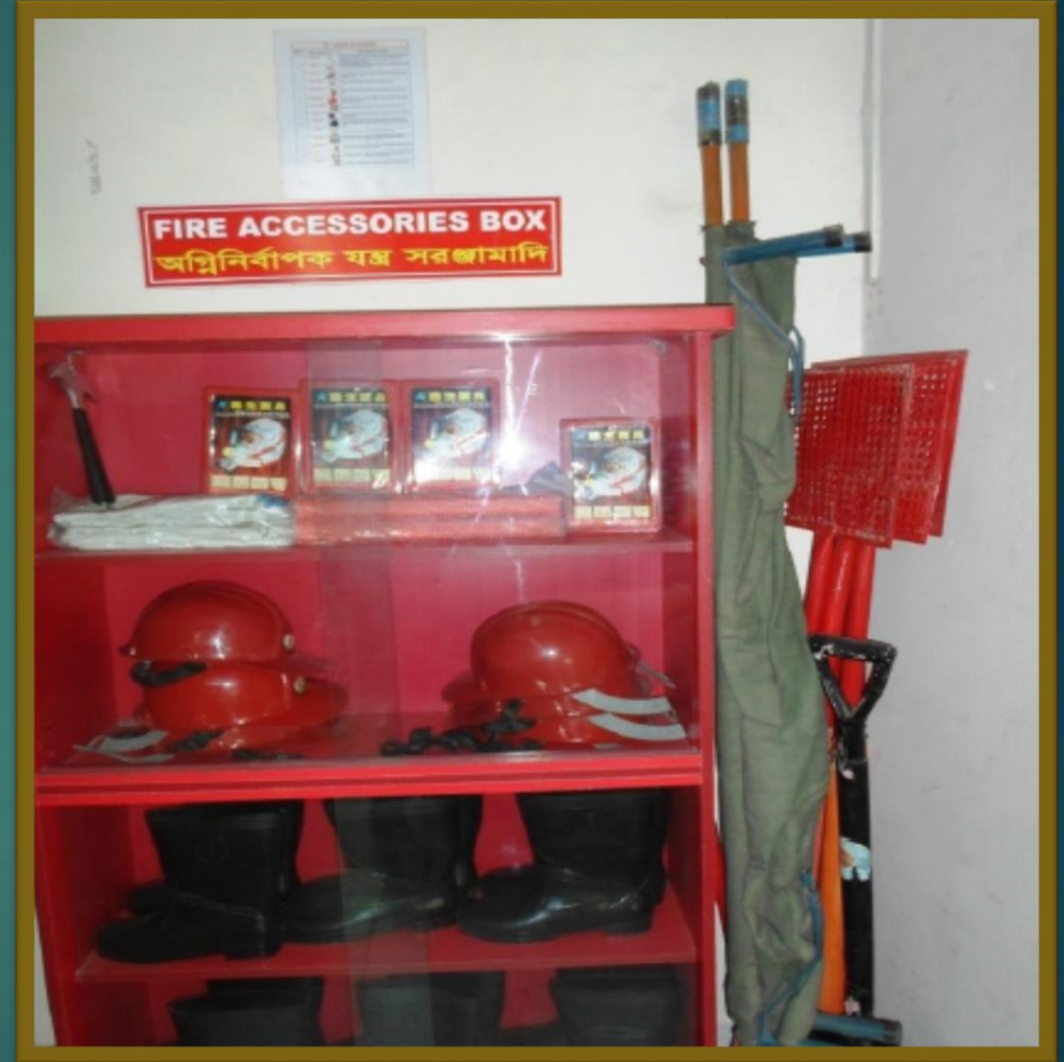
FIRE FIGHTING EQUIPMENT
